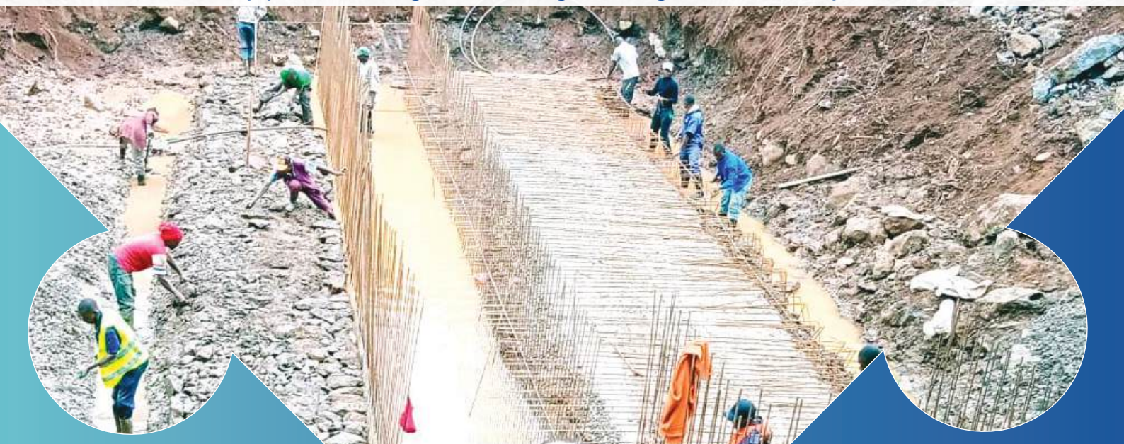
Intake Construction: Laying of blinding layer and installation of intake weir reinforcement for Kiangochi Muchungucha Irrigation Water Project in Murang'a County
