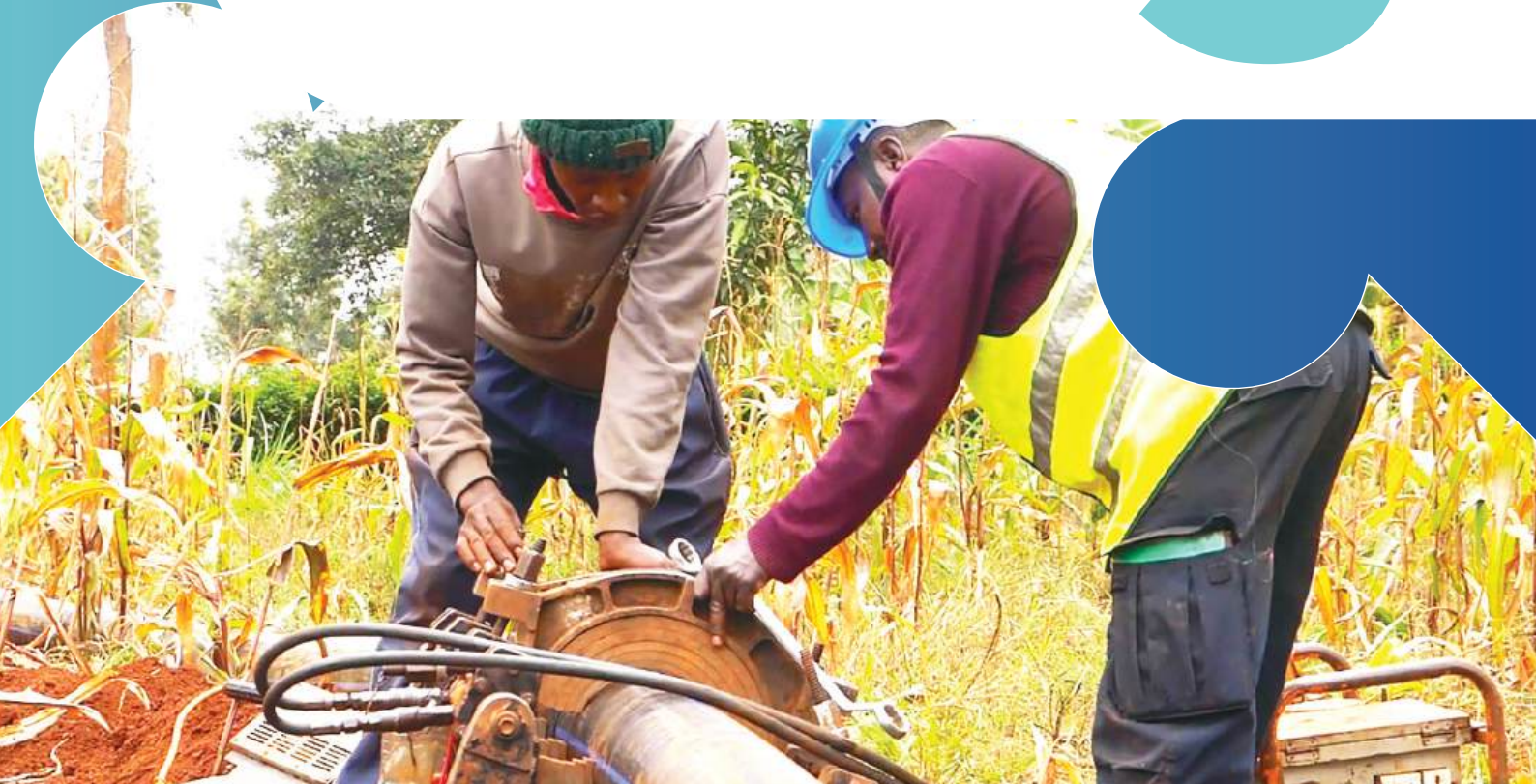
Joining high density polythene pipes (HDPE) during the laying of pipeline at Kiangochi Muchungucha Irrigation Water Project.
